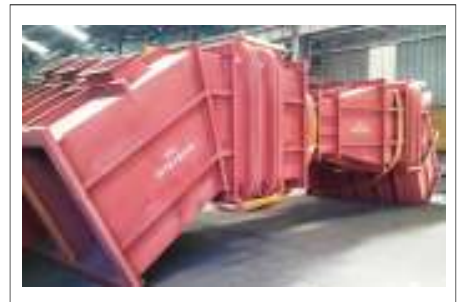
Hot Air Ducting
